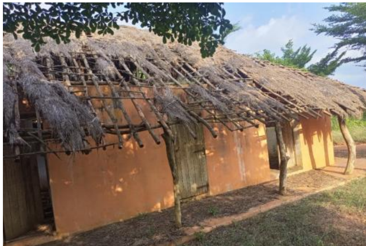
Photo No. 04: Destruction of the roof of the exhibition hall of the tourist site of the Dogbo tailed men by bad weather
